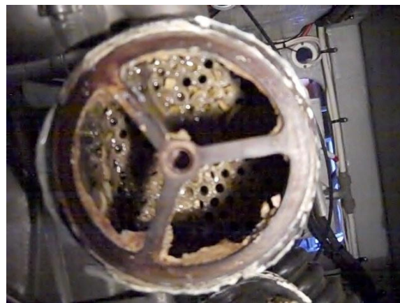
Fouled Heat Exchanger
